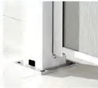
Water drainage outlet.
