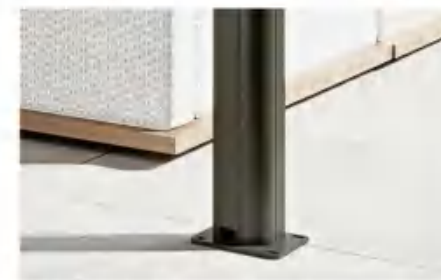
Water drop down inside the poles.
